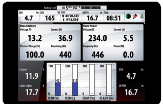
CZone installed on the Comet 45. Everyone was amazed with the remote keyfob - “Cool, I want one of those!”
